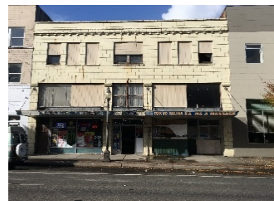
Figure 4-1. Aging downtown buildings in need of rehabilitation.
